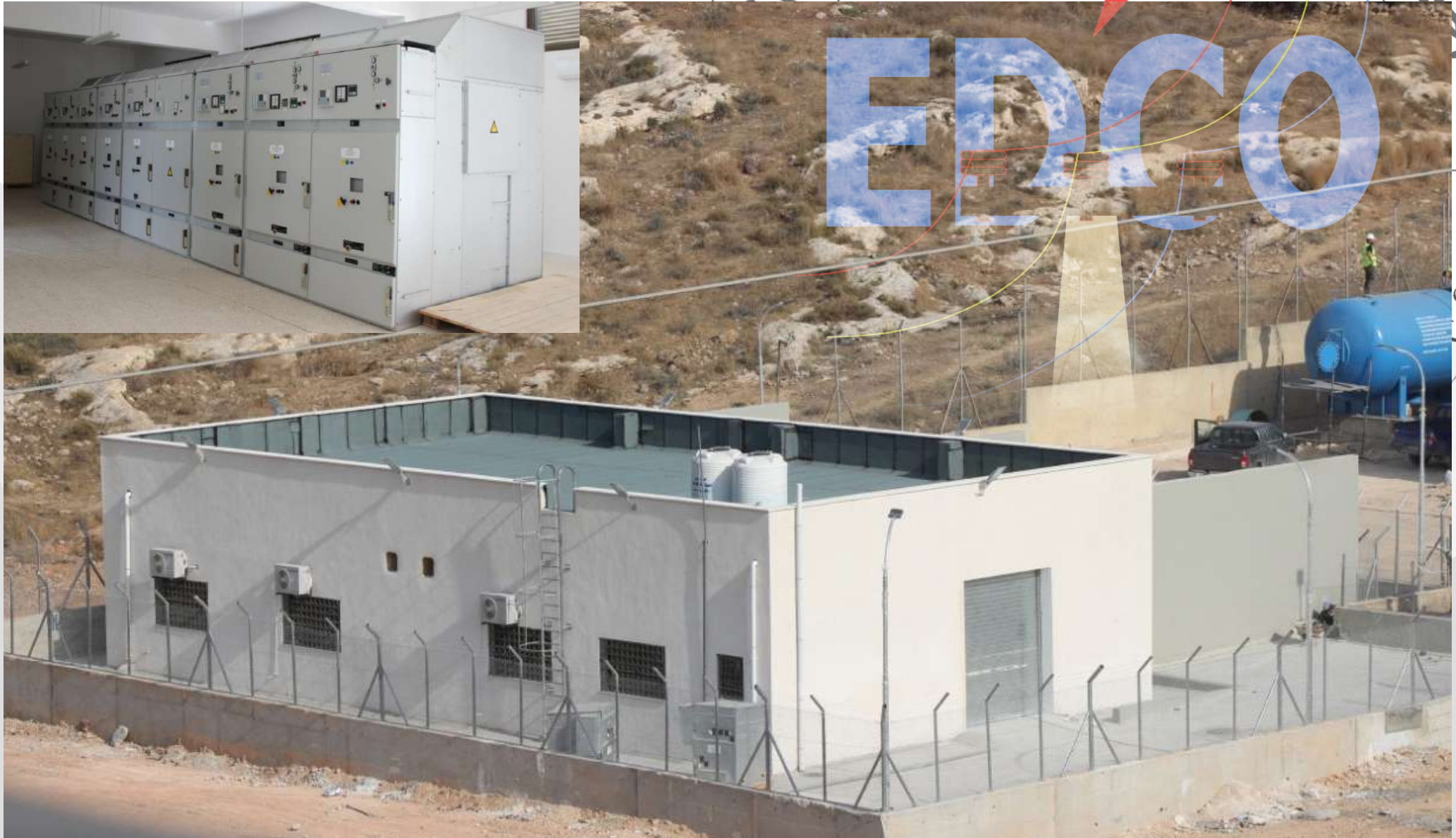
Electricity Distribution Station (PS3) Wadi Al Ordoun Dir Al Sa'na, 2019.
